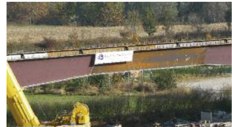
Road construction in the province of Arezzo including viaducts with about 5000 m 2 of supporting structures; here the Cantiere Morbegno
