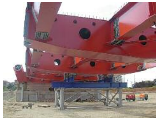
Detailed view of the bridge for the construction project of an axis of the new subterranean road network in Milan
