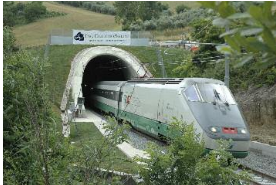
Upgrading the C shape of the Castellano Tunnel of the railway line Ancona – Varano
