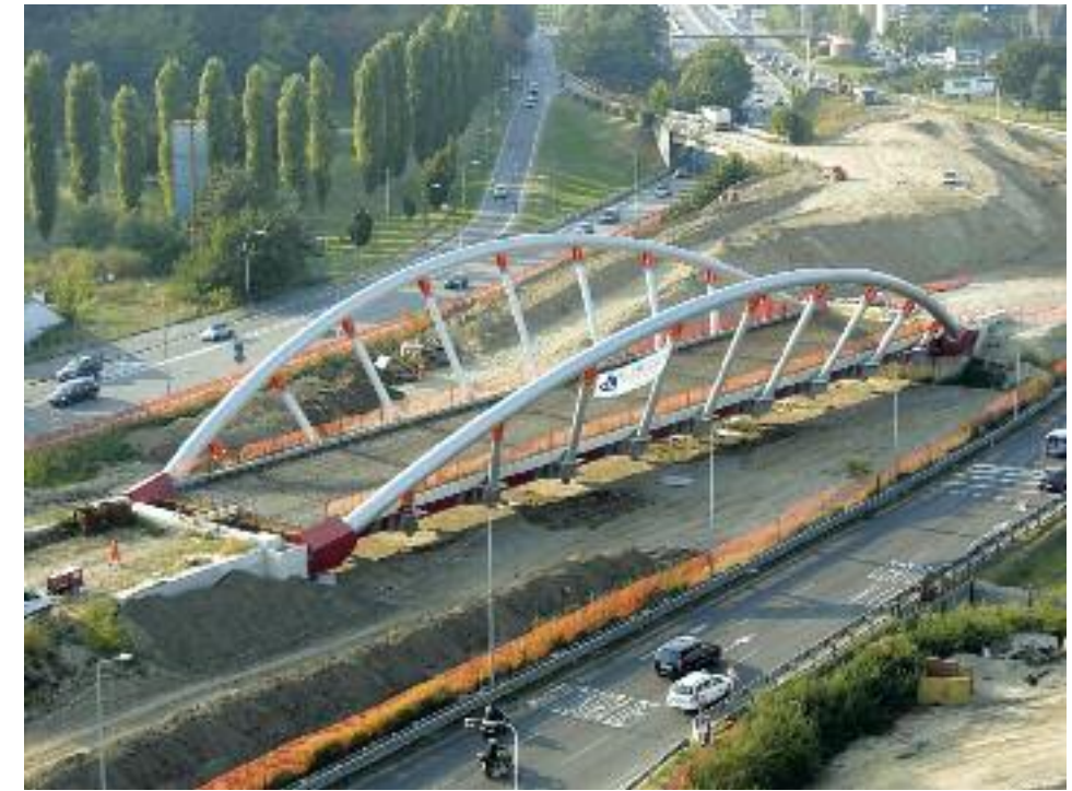
Construction of an axis of the new subterranean road network in Milan from Viale Di Gasperi to Via Gattamelata
